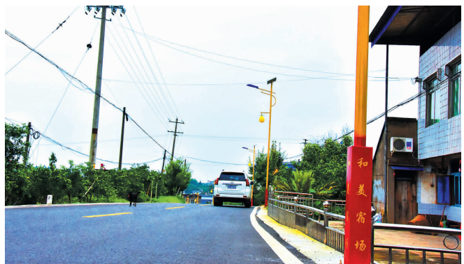
宿场村内安装的新路灯
